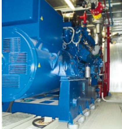
CHP unit of a biogas plant
