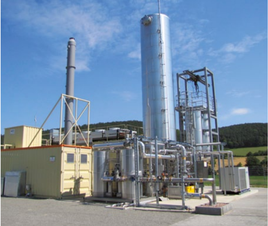
Biogas upgrading plant
