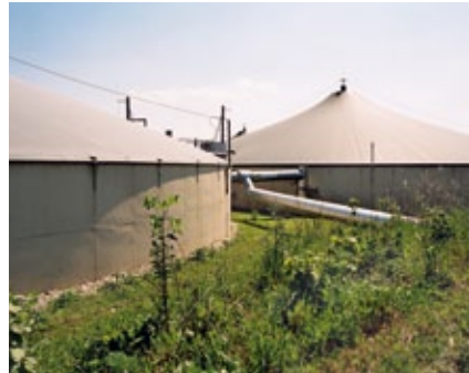
Through-flow installation with foil hood as integrated gas storage
